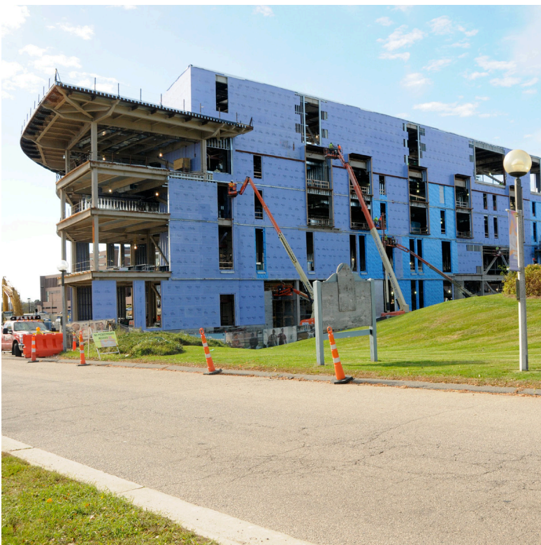
The General Academic Building No. 1 is being enclosed for indoor construction during the winter. Opening is scheduled for fall 2015.
