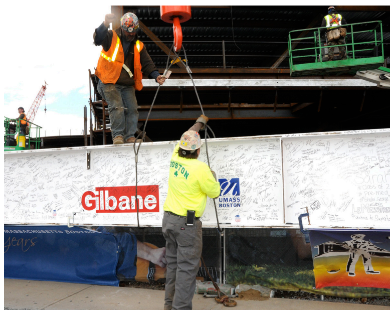
Local 7 ironworkers prepare to hoist the final steel beam, covered with signatures and well wishes from the UMass Boston community, atop the frame of the GAB No. 1.
